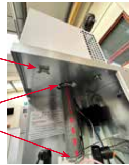
View from the inside of the Vapac Unit showing RDU in situ
