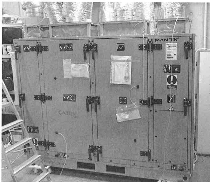
Fig. 2 Air handling unit during measurement
