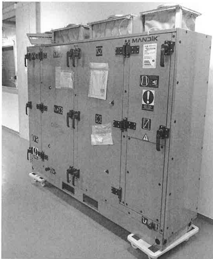
Fig. 1 Tested air handling unit
