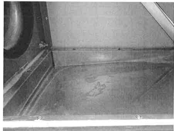
Fig. 10 The space between the heat exchanger and the fan on the exhaust air side
