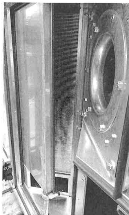
Fig. 12 Exchanger, bypass, condensate drain and fan
